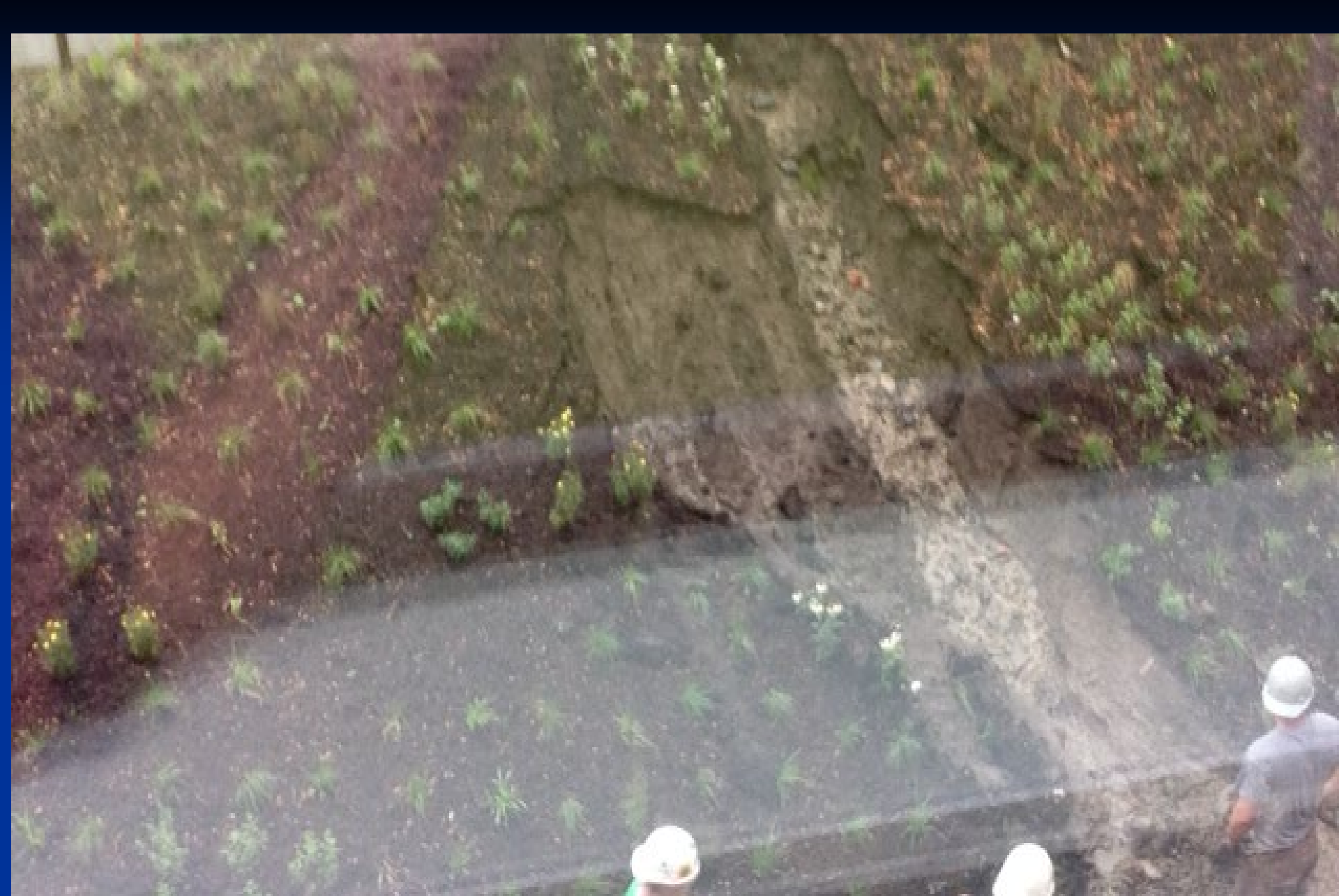
Slope failure -blanket was improperly built
